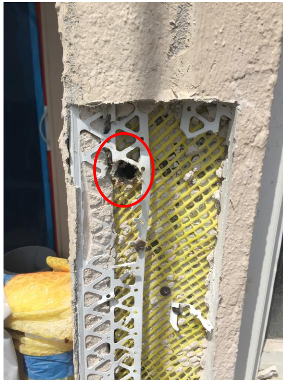
Picture 4: Fastener hole from shutter that will need to be repaired
